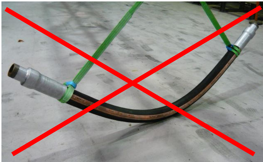
Figure 10: Incorrect installation of hose (touch down effect) The hose is subjected to abrasion over bending and undue stresses in the hose body (i.e. compression)
